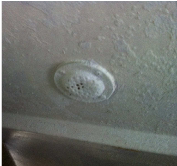
Figure 1: Partially blocked skin fitting grille
